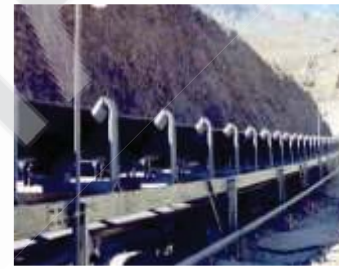
Fig. 15 – Primary crusher of the conveyor system Minera Los Pelambres [19]
