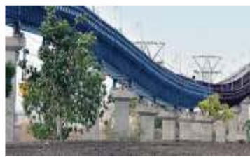
Fig. 20 – Conveyor system Heidelberg Cement, Damoh [21]
