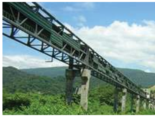
Fig. 10 – Conveyor system in Bangladesh [6]
