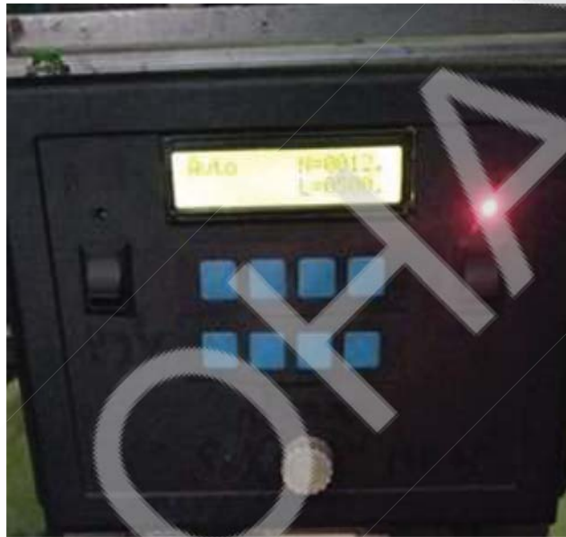
Picture 18 – The control unit
