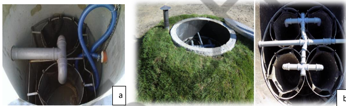
Fig. 14. Installation for dewatering and disposal of sewage sludge. a- in Florianka in the Roztocze National Park, b- in Stare Załucze in the Polesie National Park
