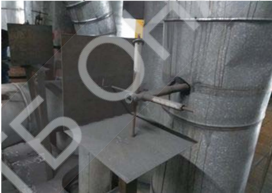
Fig . 1. Mechanical indicator of thermal displacement of steam lines
